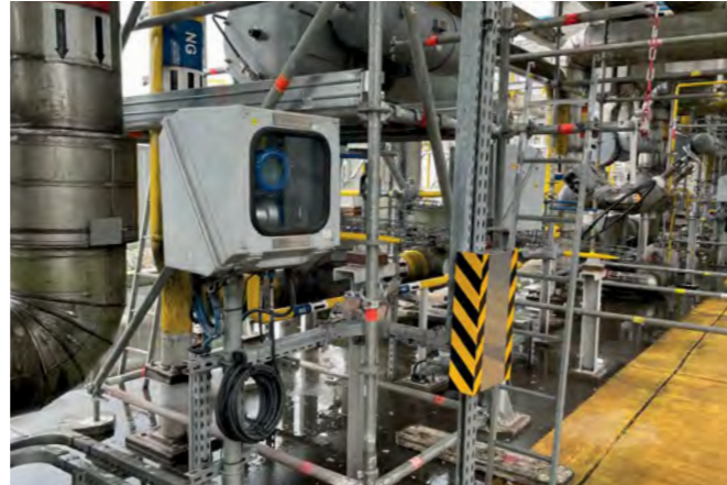
Temperature controlled transmitter enclosure for LNG terminal.
