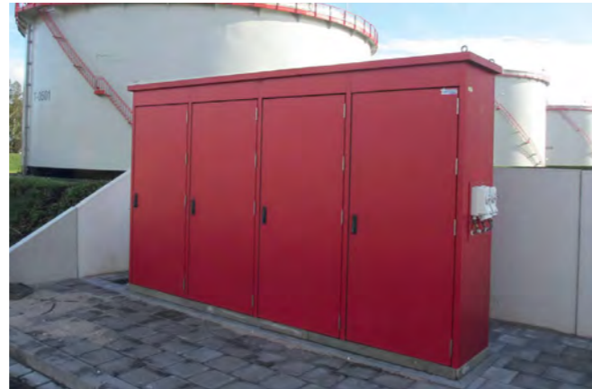
Fire fighting equipment.
