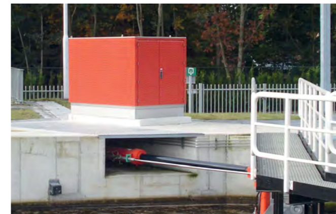
Multi-compartment cabinet for electronics and hydraulic systems controlling a waterway lock.
