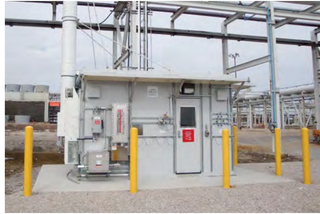
Continuous Emission Monitoring System shelter for a flare stack at a chemical processing plant.
