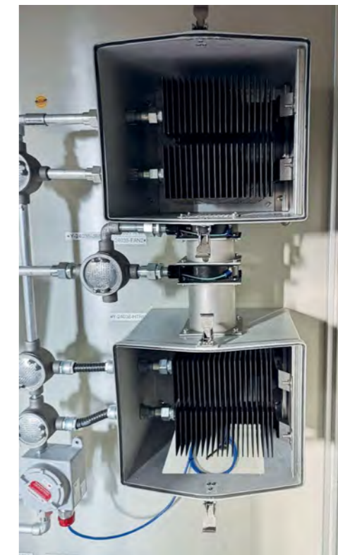
Redundant ventilation fans with pre-warming system.
