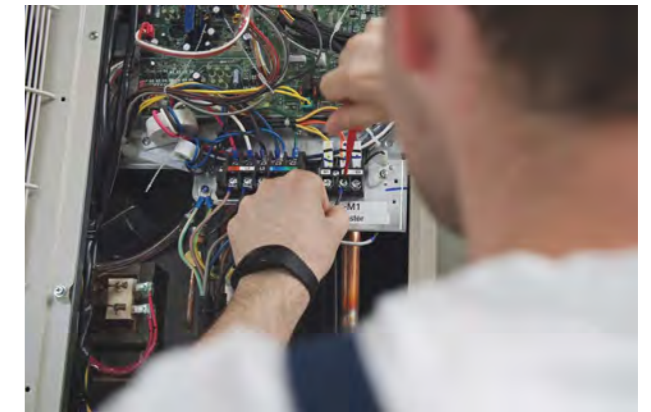
All wiring is done in-house by qualified electricians.
