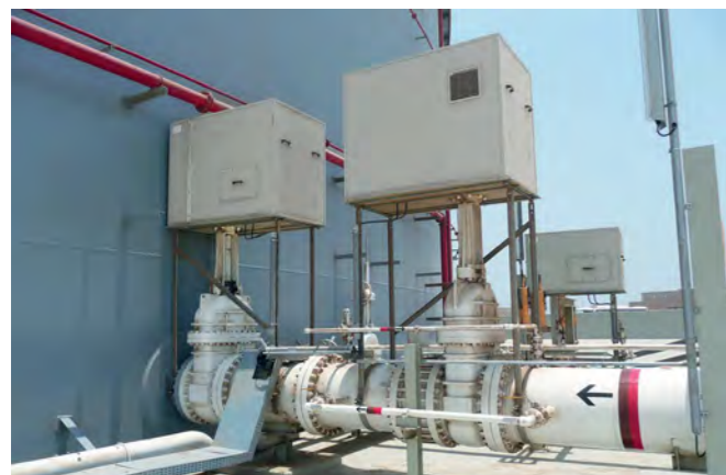
FIRE SHELTERS protecting emergency shut-down valve actuators.
